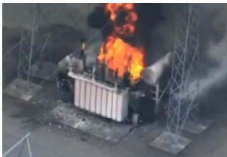
Fig. 2. Example of transformer failure with fire
